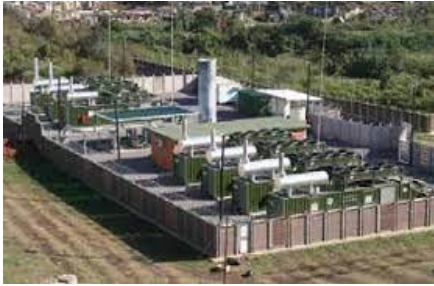
Landfill gas to electricity
