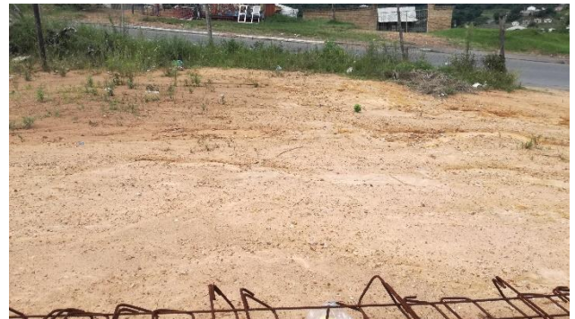
Figure 27 | Erosion caused by the lack of vegetative cover and energy dissipating measures north of erf D
