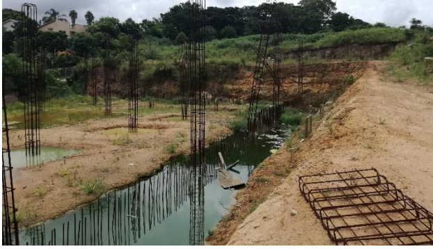
Figure 24 | Column reinforcement rebar protruding from excavations, posing a fall- and drowning risk
