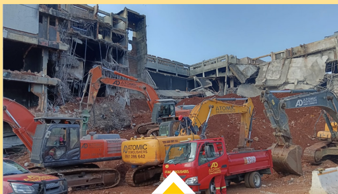
The mechanical demolition of the China Emporium is proceeding well and is expected to be complete by September.
